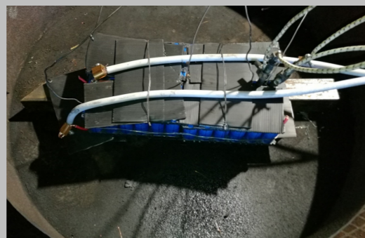
Battery pack power connecting wiring glow plugs
