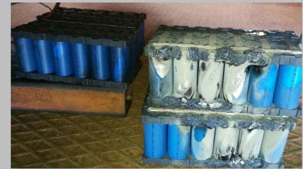
Battery cells aggregate after extinguishing/ controlling the runaway
